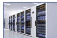
Data Centers & IT Facilities
